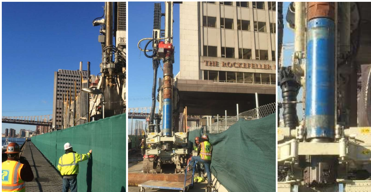
Figure 7. Maintaining vehicular traffic on the FDR Drive and pedestrian traffic on the esplanade, shown at left, while rock drilling with air-flush required planning and constant vigilance to prevent property damage and injury to the public. The Roto Loc under-reaming system can be seen in the photo on the right.
