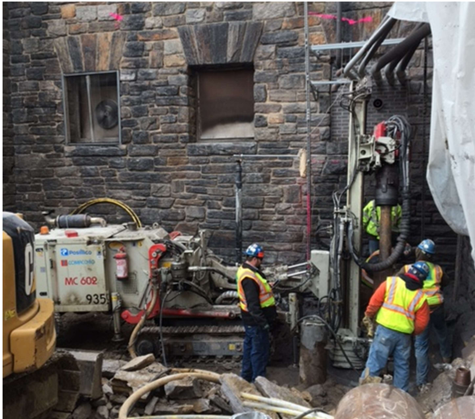
Figure 7. Construction of MER A foundation was performed with small rigs within tight constraints. The photo shows the installation of mini-caissons battered 1 on 4 (horizontal to vertical). Also shown, upper right, are the active electrical ducts just above the drill rig mast. The headroom restrictions required the use of 5-foot long casing and drill rods.
